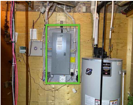
Basement Mechanical Room
