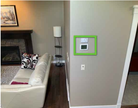
Thermostat: Start of Inspection
