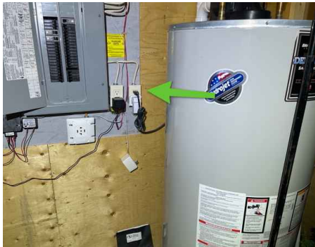
Water Heater Shutoff: Electrical Shut Off Location Left Side of Water Heater
