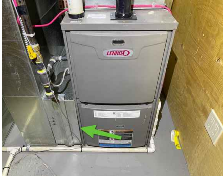
Heating System 2: Filter Left Side of Heating System
